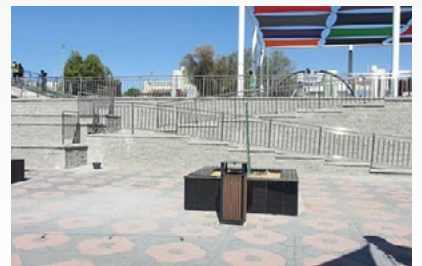
Flexibility of the TensarTech TW1 ME wall system enabled access ramps to be easily incorporated into the design.
