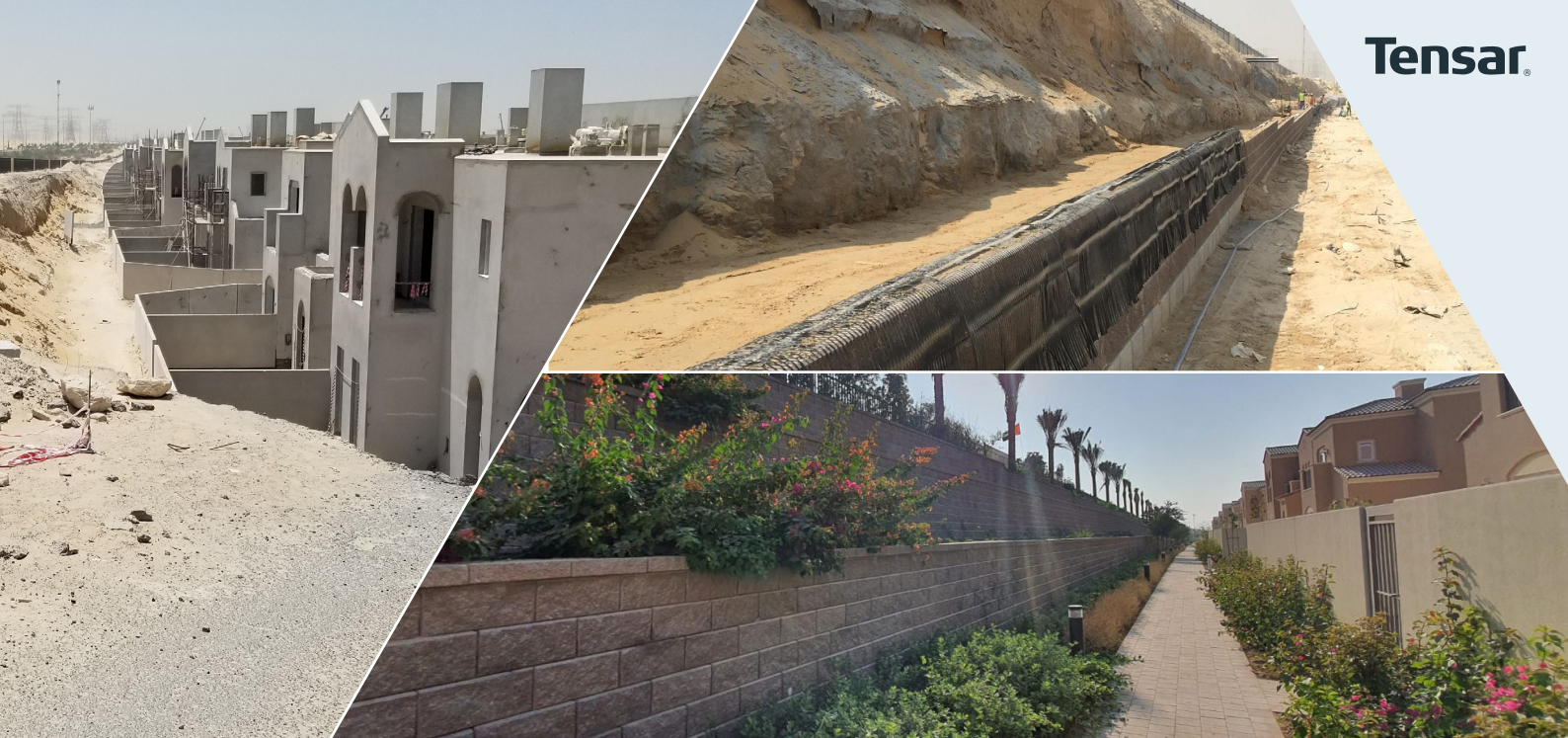
TensorTech TW1 ME Wall before construction (left), during construction (top right) and after construction (bottom right)
