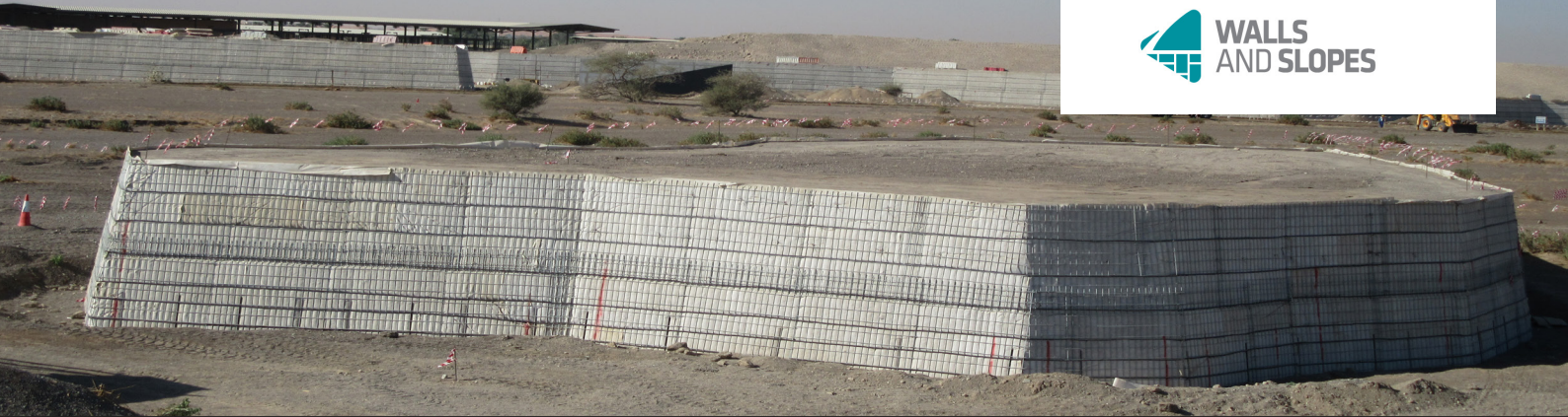
TensarTech TR2 reinforced soil wall system was chosen to form the raised 'islands' to create landscaped animal enclosures
